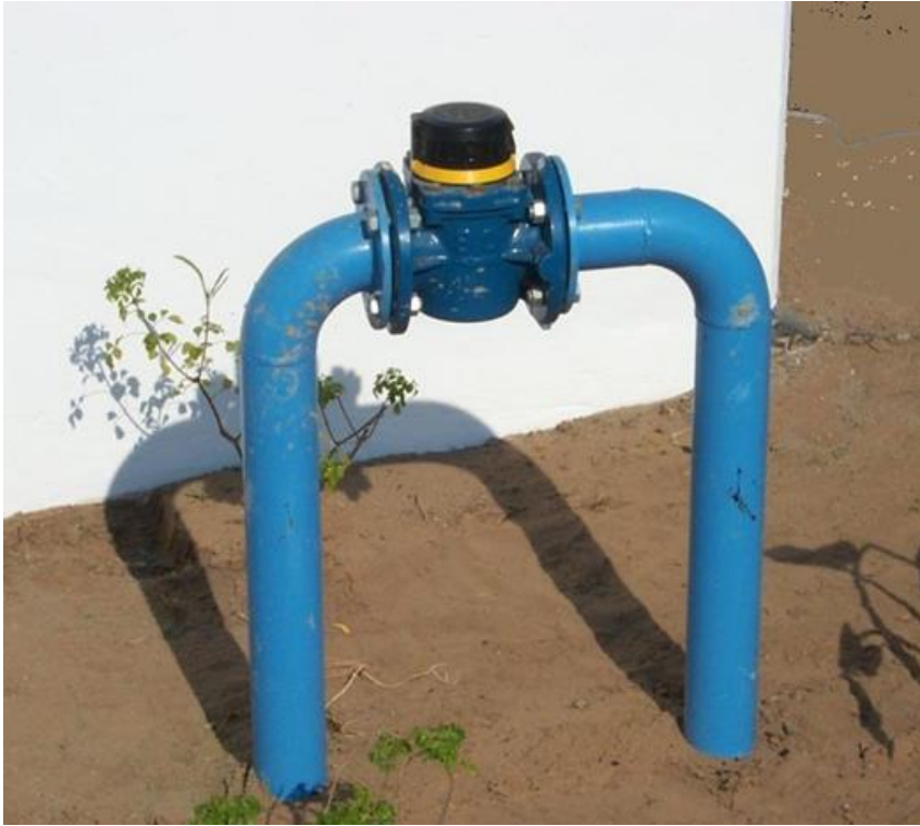
Insufficient straight pipe – Perfect air trap
