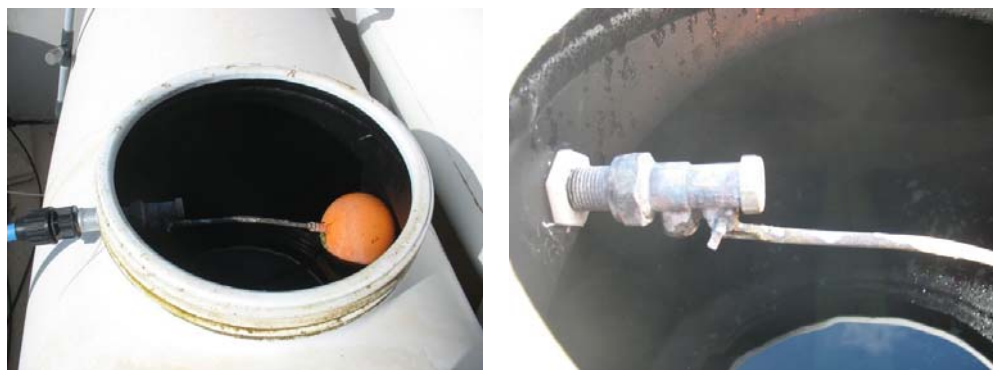
Figure 4. Polypropylene Roof Tank
